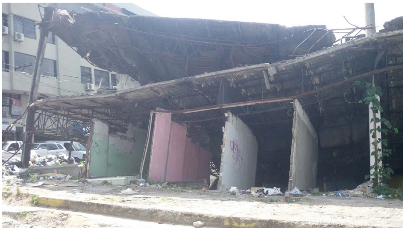
San Cristóbal, Venezuela. Much of the infrastructure has been looted and burned. (Fox News/Hollie McKay)
